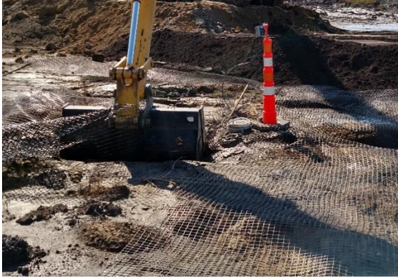
Figure 3: Access Road Underlain By Failing Soft Layer
